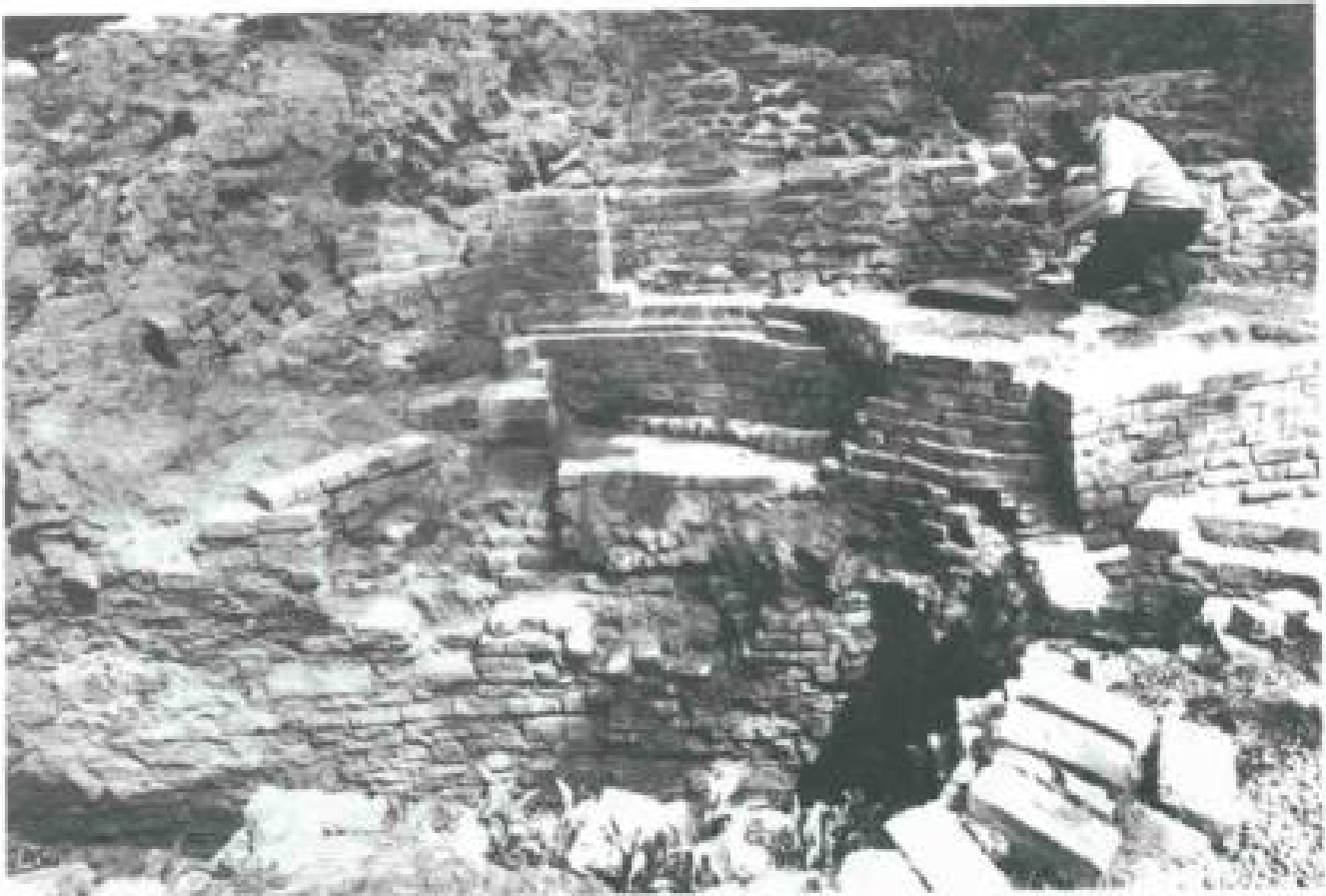
Restoration in progress to western wall of Pumphouse and to the Haystack boiler setting.
