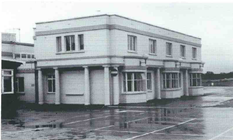
Fedden House (K), from north-west, building 306A (T) extreme left, immediately prior to demolition (7 October 1995).
