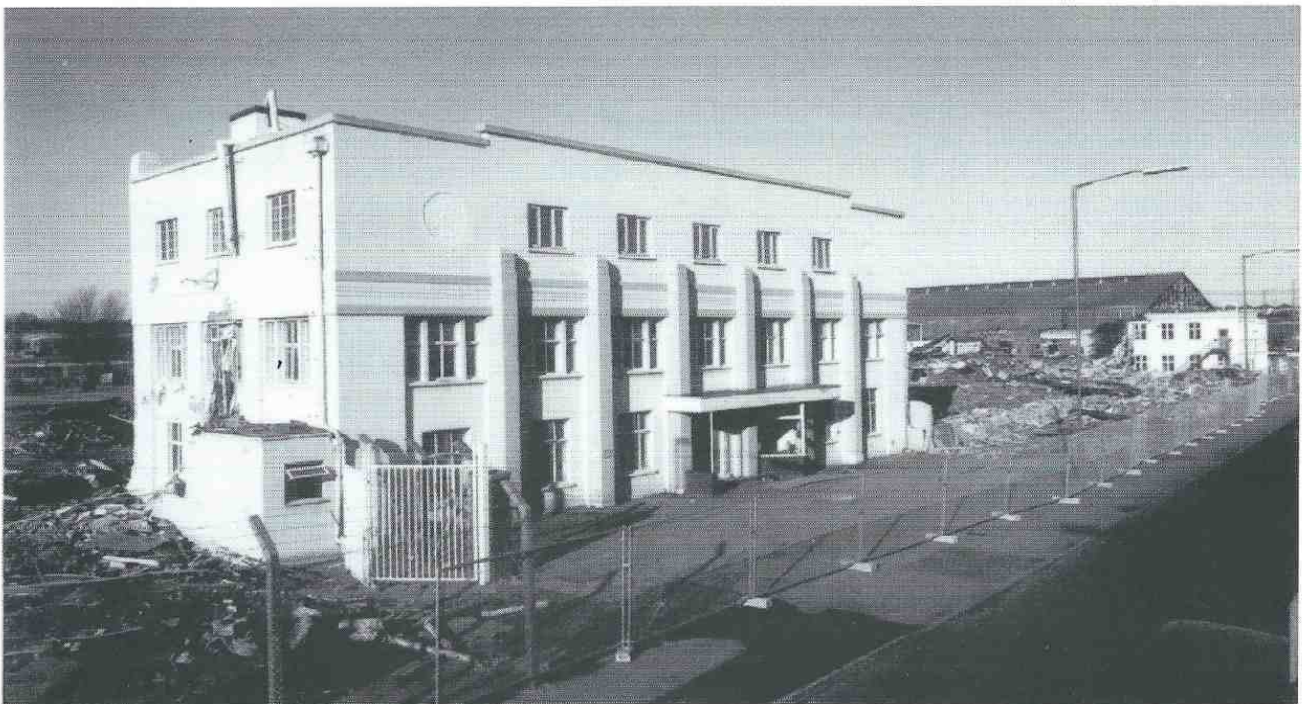
Former engine HQ building (D on plan) from south-east, during demolition (2 November 1995).
