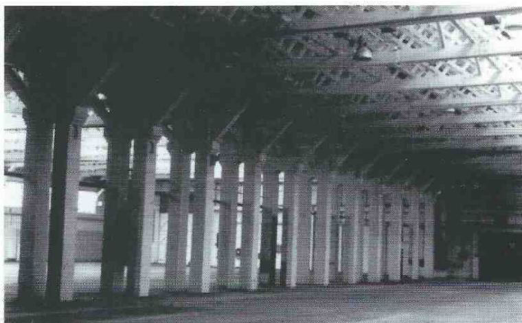
Right, Interior of centre hangar (B) showing roof trusses and original arrangement of brick piers (7 October 1995).
